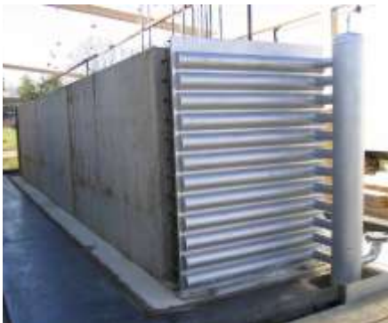
▪ Concrete storage module without insulation
