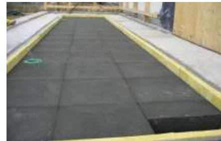
▪ Concrete storage module with insulation
