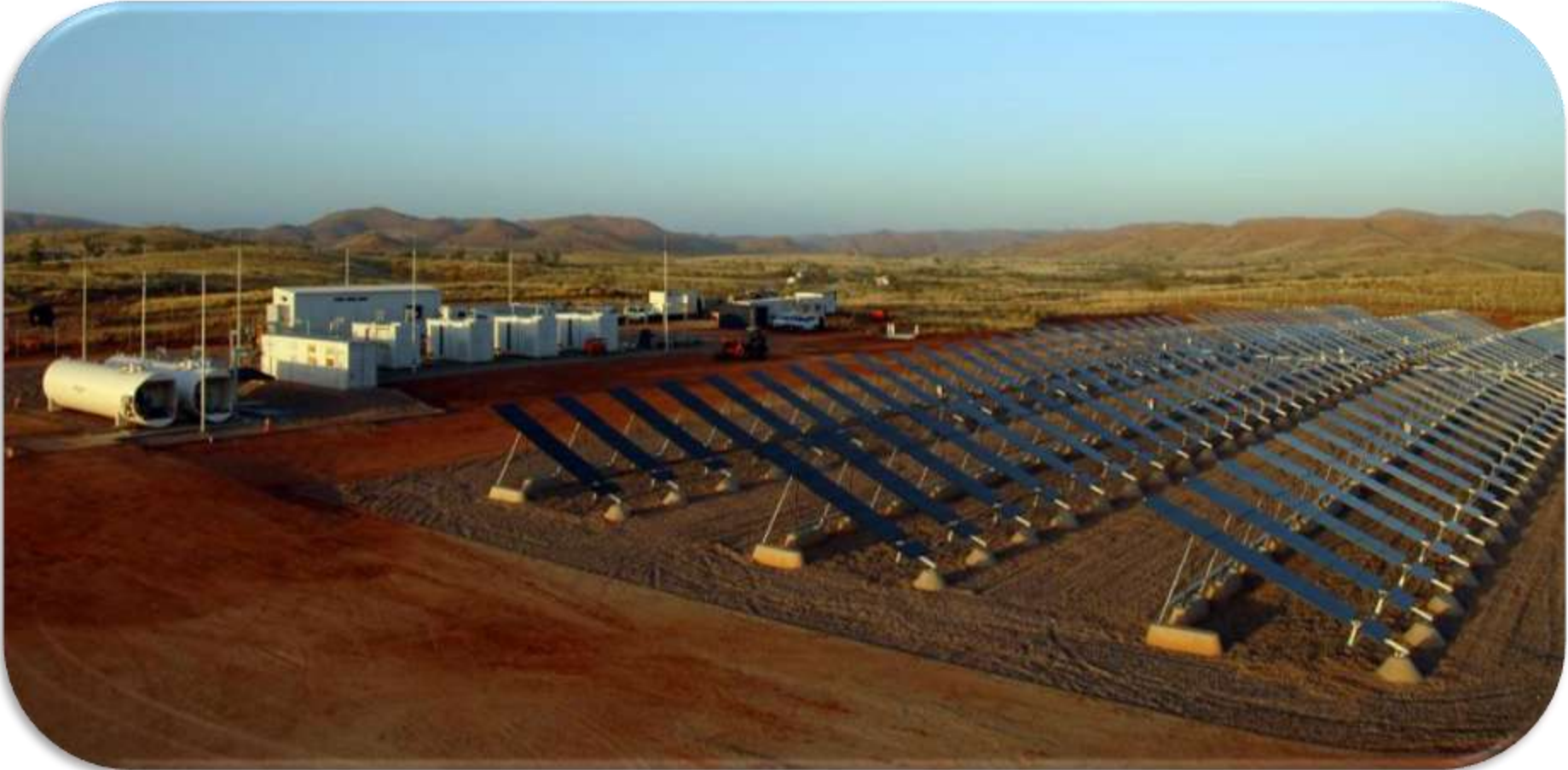
Marble Bar Solar/Diesel power station, Western Australia
